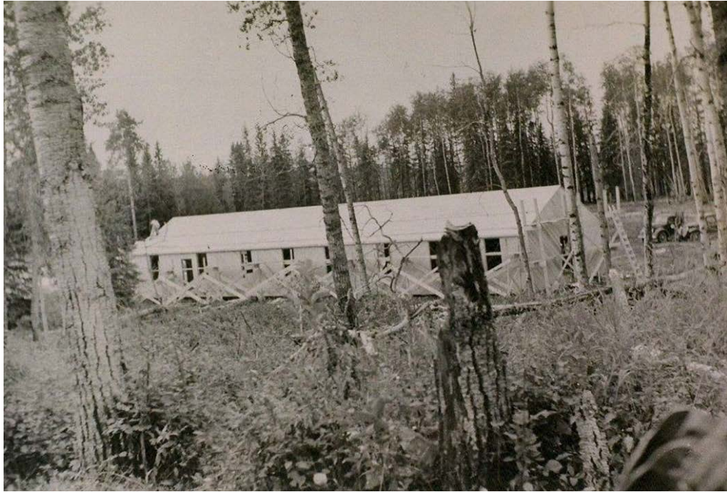
Figure 8.14: Riding Mountain Camp guard barrack structure under construction in October 1943. (Courtesy of Pinewood Museum)
