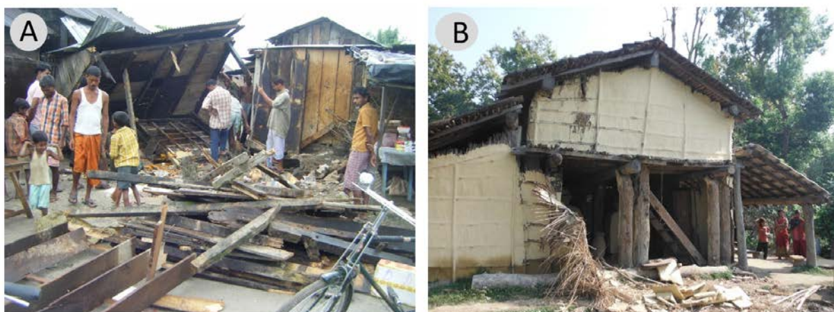
Plate 1: Property damages caused by elephants in search for food (A) in MA to a grocery store at Gadulee Market in May 2009, Bansbari, and (B) to a farmhouse in BA at Suryapatuwa in May 2009, the entire wall has been removed by the elephant, clearing the view on traditional rice storages on the ground floor.
