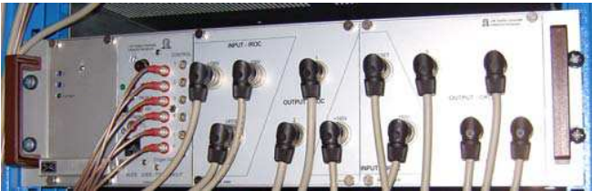
Abb. 6: ALICE Gating Grid Pulser System Patchpanel V1.1
