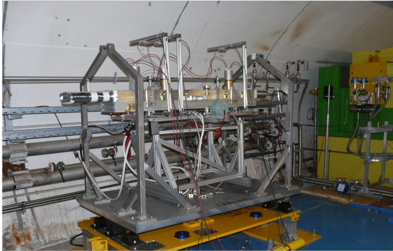
Fig. 6.5: Hydrodynamic tunneling experiment installed in the HiRadMat facility. The dBLMs are mounted on the three aluminum arms on top of the experimental setup.
