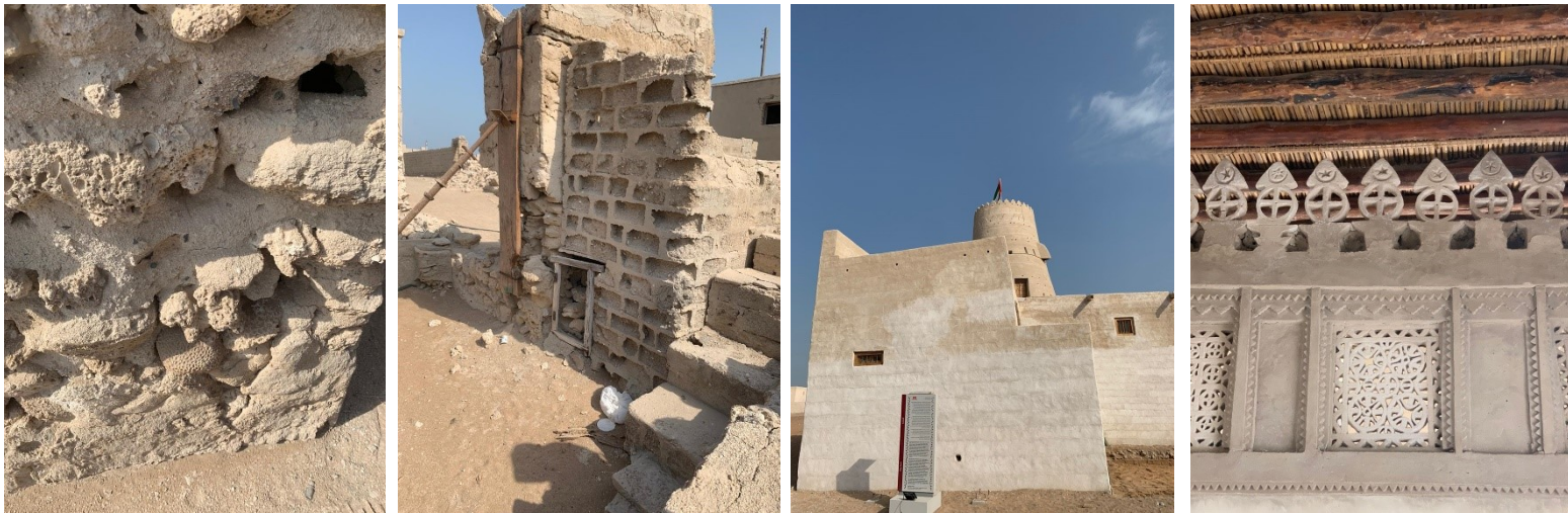
(from left to right) The use of coral and beach rock, The introduction of cement, The fort, Intricate original reliefs made of gypsum in one of the houses in JAH
