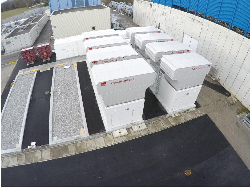
Figure 5.2: CR0 Data Centre view after two IT-Containers were installed at Point 2.
