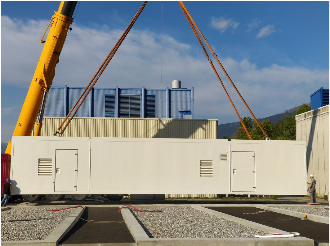
Figure 5.1: Installation of the power and utility container at P2 as the first step of the Data Centre installation in 2018.
