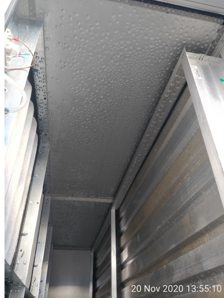
Figure 6.20: Condensation inside an offline cooling unit when operating with two out of four units at a low load scenario during cold weather conditions.
