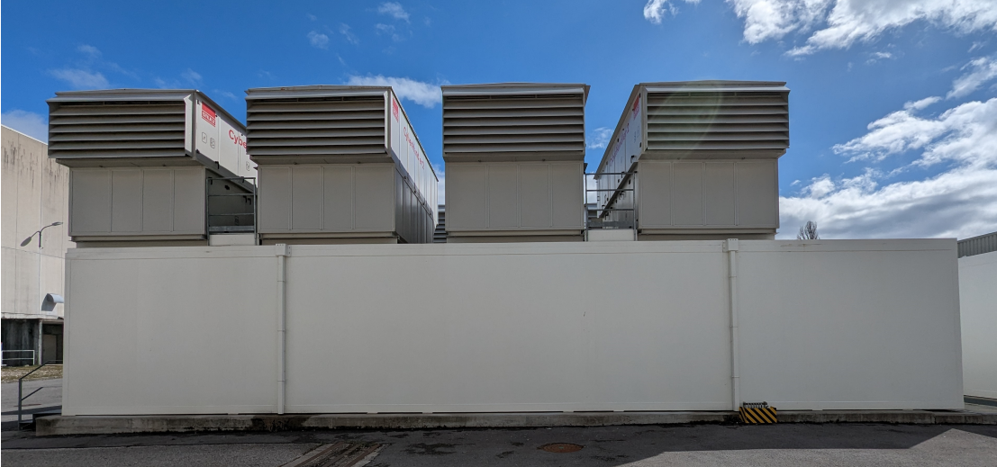
Figure 5.5: IT Container with 4 cooling units side view.
