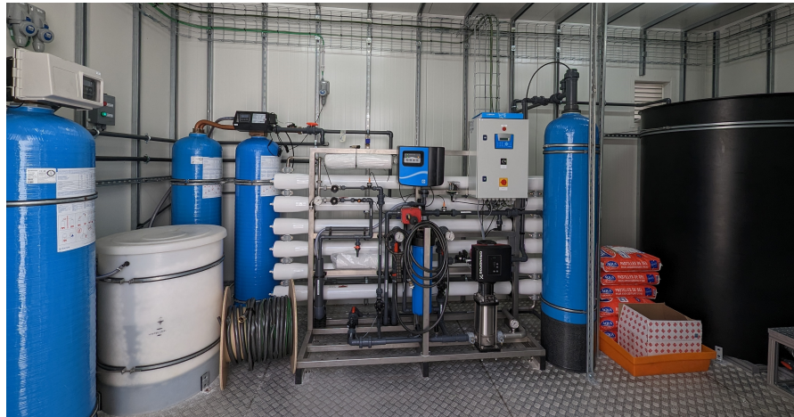
Figure 5.10: Water treatment installation in the infrastructure container. The leftmost blue bottle is an activated carbon filter, to remove chlorine. Next to it is a salt reservoir for the softener stage (two blue bottles), replacing calcium and magnesium with sodium ions to protect the reverse osmosis membrane. In the center of the picture there are six reverse osmosis tubes, filtering large particles from the water. Small buffer tank (blue) to the right provides clean reverse osmosis water to clean the membranes. Big black buffer tank to the right keeps approximately 2000 L reverse osmosis water for the cooling units.
