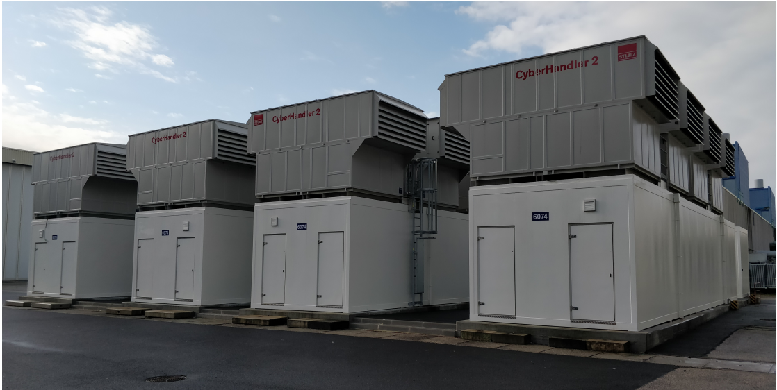
Figure 6.1: Fully assembled Data Centre at P2, with 4 IT-Containers in place. The total cooling capacity of 2.1 MW split equally between the 4 containers. 250 EPNs are housed in IT1 and IT2, the two rightmost IT-Containers in the picture [14].
