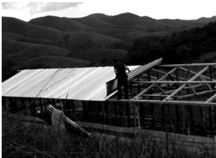
The roof of the primary school in Murhume, Nindja, is covered with metal sheets. This construction was funded by a donation from the Dutch bank Kempen & Co.
