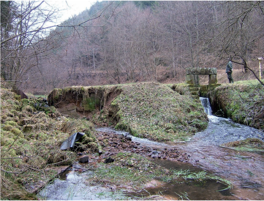
Fig. 9: Drift pond dam from the 19 th century with historical outlet structure (right side) and damage requiring restoration (left side).
