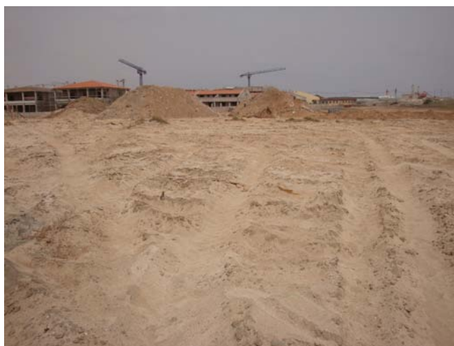
Fig. 15. Compaction of sand due to construction traffic on Algodoeiro.
