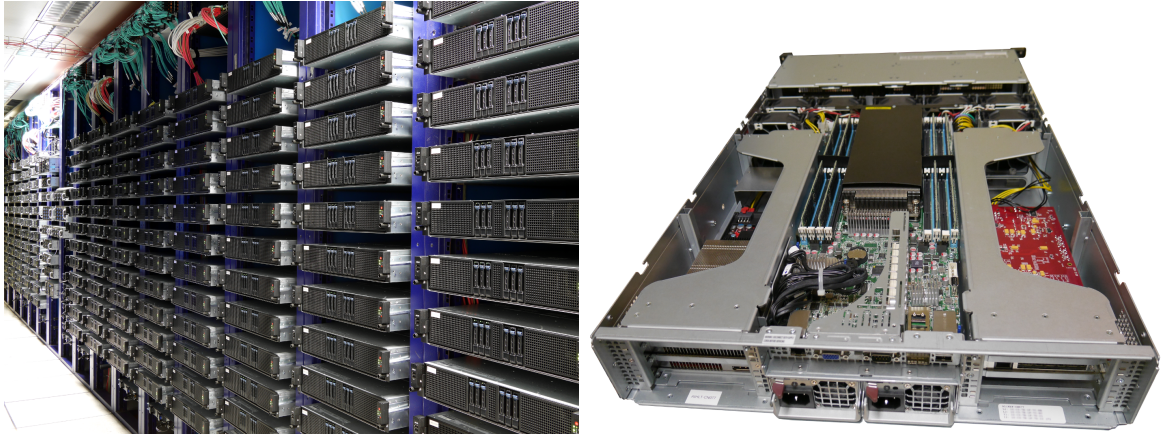
Figure 3.2: Left: Photo of the ALICE HLT at start of RUN 2. Right: interior of a node. The GPU is installed in the left tray, the C-RORC in red on the right.
