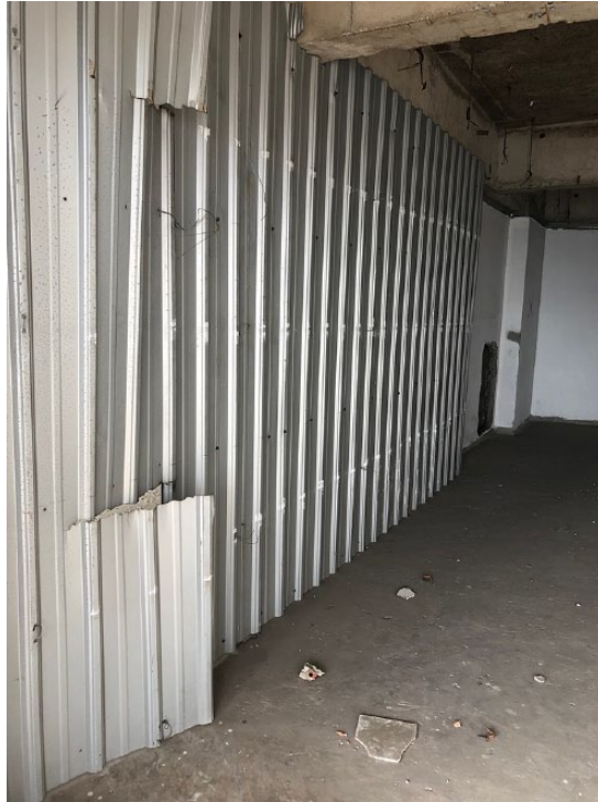
Figure 3. The cause of the noise on the 27th floor of the Ghost Tower.
