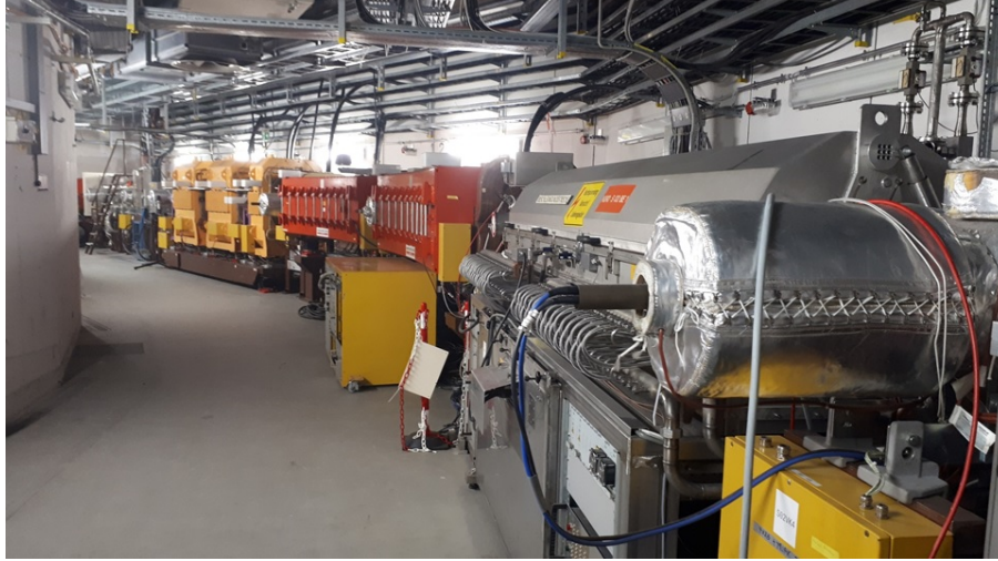
Figure 2.1 One section of SIS18 hadron synchrotron showing the RF cavity, two dipole magnets and three quadrupole magnets.
