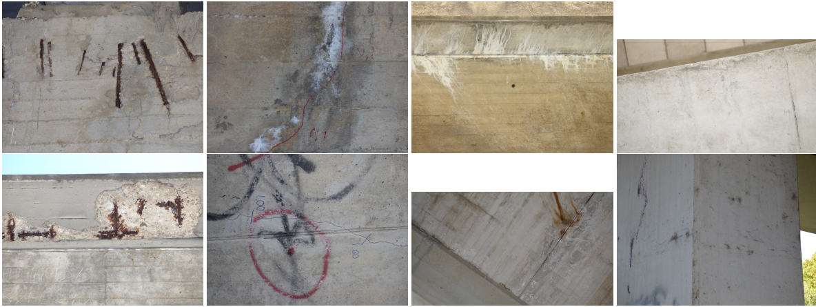
(a) Top row from left to right: 1.) exposed bars, spallation, cracks (hard to see) 2.) hairline crack with efflorescence 3.) efflorescence 4.) defect-free concrete. Bottom row from left to right: 1.) large spalled area with exposed bars and corrosion 2.) crack with graffiti 3.) corrosion stain, minor onset efflorescence 4.) defect-free concrete with dirt and markings.
