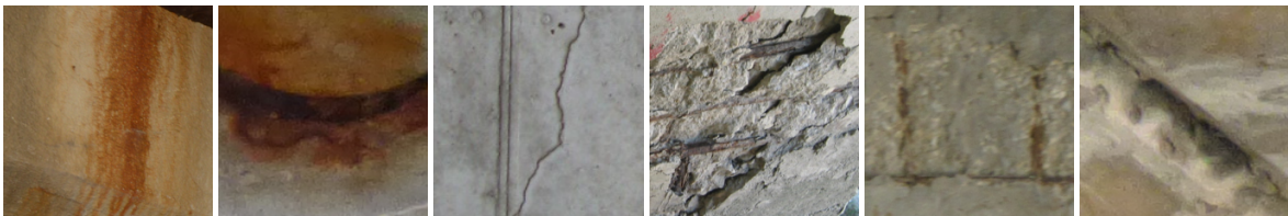
(b) False multi-target classification examples from the validation set where at least one present defect class is recognized correctly. From left to right: 1.) corrosion (predicted corrosion and efflorescence). 2.) corrosion (predicted corrosion, spallation and exposed bar). 3.) crack (predicted crack and efflorescence). 4.) spallation, exposed bar, corrosion (predicted spallation and corrosion). 5.) spallation, exposed bar, corrosion (predicted crack and corrosion). 6.) efflorescence (predicted efflorescence and crack).
