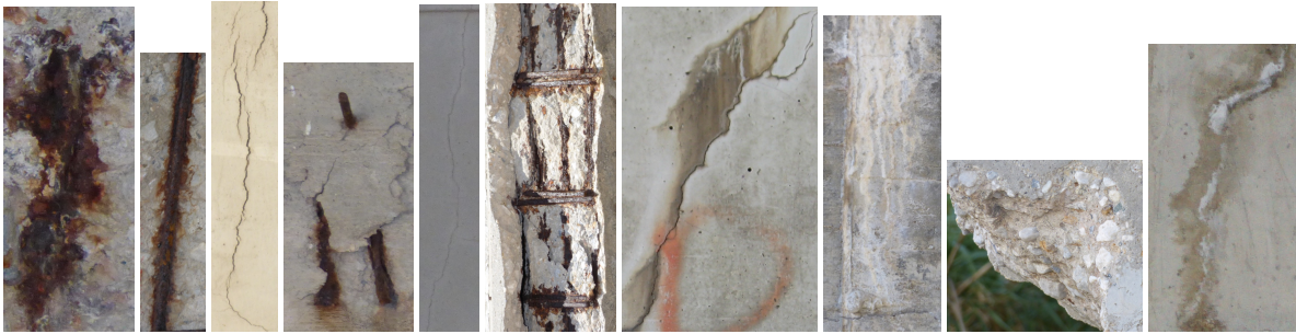
(b) From left to right: 1.) spalled area with exposed bar, advanced corrosion and efflorescence 2.) exposed corroded bar 3.) larger crack 4.) partially exposed corroded bars, cracks 5.) hairline crack 6.) heavy spallation, exposed bars, corrosion 7.) wet/damp crack with efflorescence on the top 8.) efflorescence 9.) spalled area 10.) hairline crack with efflorescence.
