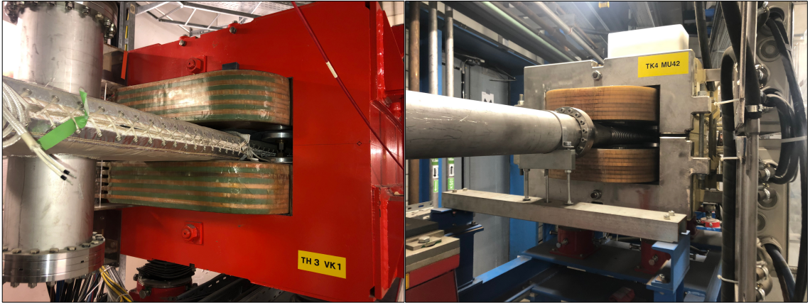
Figure 2.7.: Two examples of brick shaped dipole magnets. (left: GSI high energy transfer line, right: transfer channel TK to SIS18)
